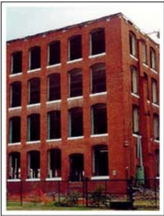
Building without the character-defining element, historic wooden windows
